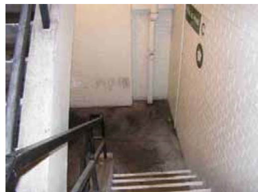
Photo 7: Non-refurbished stairwells at multi storeys
